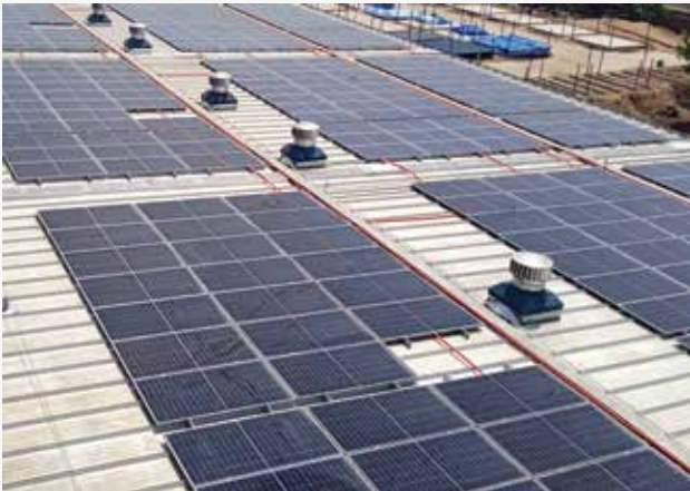
Solar Plant at Cuttack
