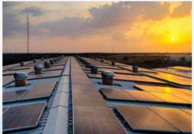
Solar Plant at Halol Composite
